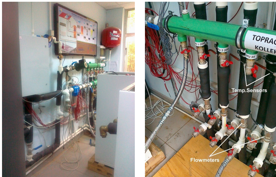
Figure 6. Thermal response test system.
