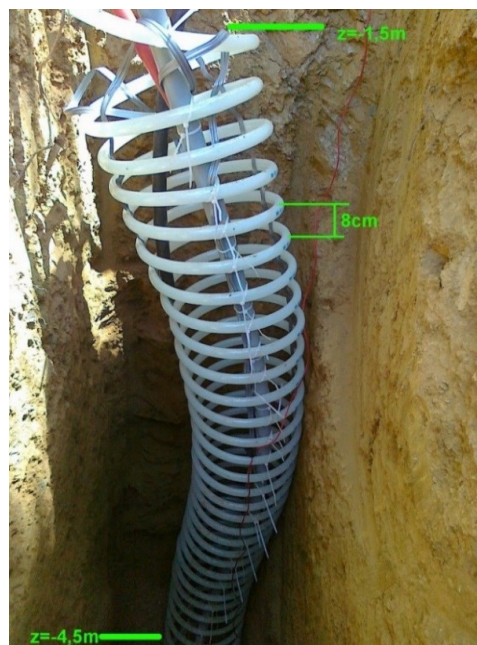
Figure 4. Vertical Helix GHEs in application field of Energy Institute-ITU/Istanbul/Turkey.
