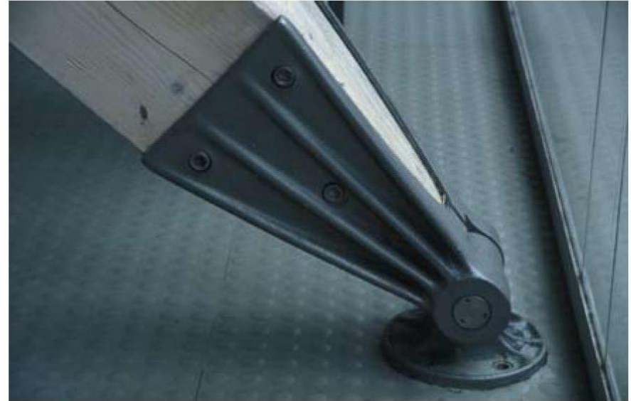
▲ 7.30 Lyons School of Architecture, France, Jourda et Perraudin, 1988. A cast-steel shoe expresses the compression load-path.
