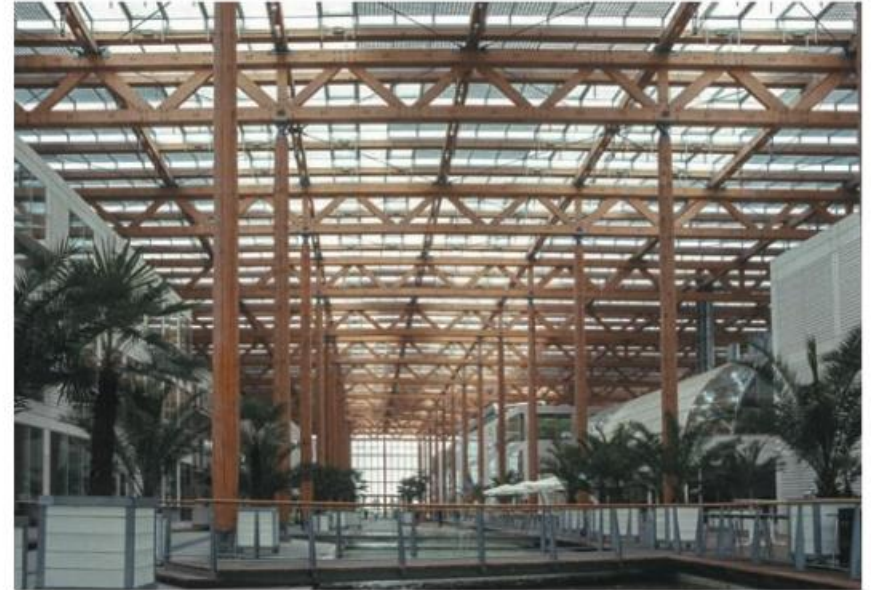
Figure 3.3 Post and beam gravity structure. The beams, detailed as trusses, are continuous over several spans.
