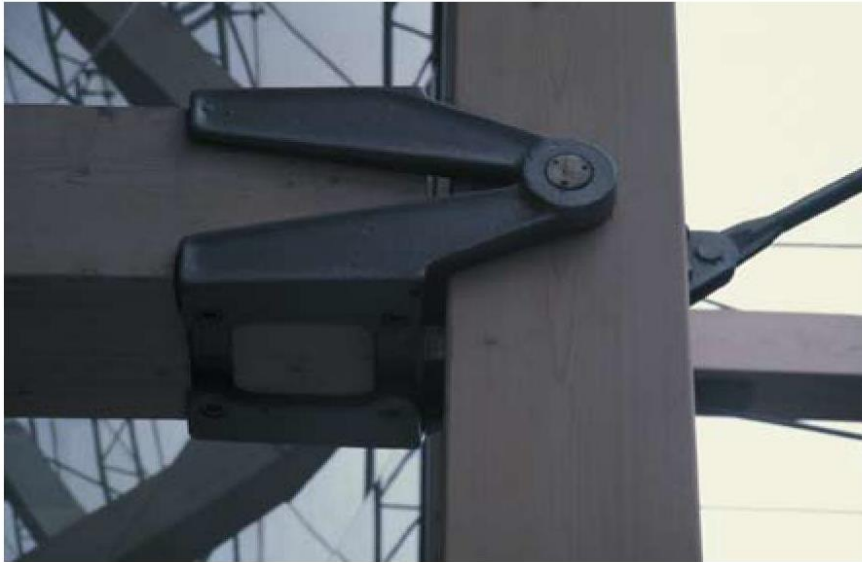
▲ 7.31 A beam-column connection where a horizontal gap between the castings allows for a down-pipe to pass through the detail where required.
