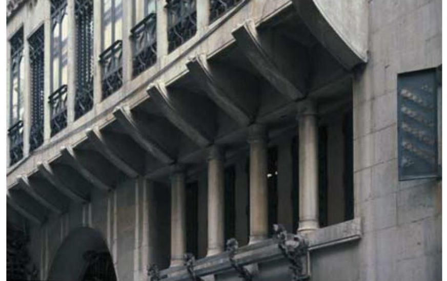
▲ 7.32 Palau Güell, Barcelona, Spain, Antonio Gaudí, 1880. Cantilevering brackets clasp the oriel floor.
