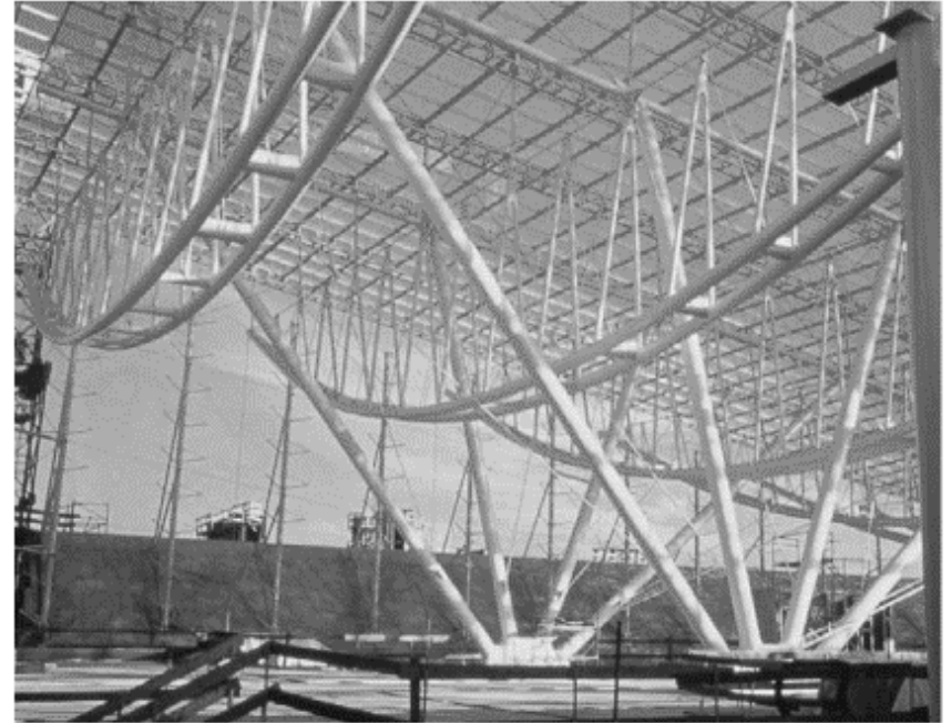
4.41 Deep curved roof trusses at the TGV terminal at Charles de Gaulle Airport, Paris (architect: Aeroports de Paris)
