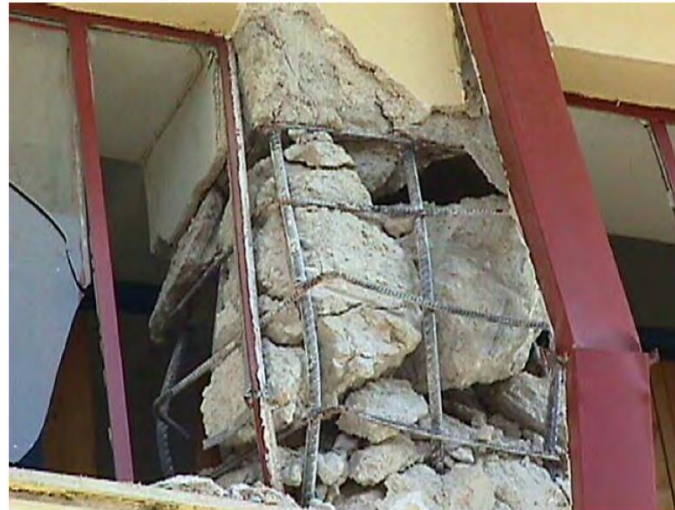
Failure of a column dimensioned according to old regulations that required a peripheral stirrup with its end bent in 90° instead of 135° (45°).
