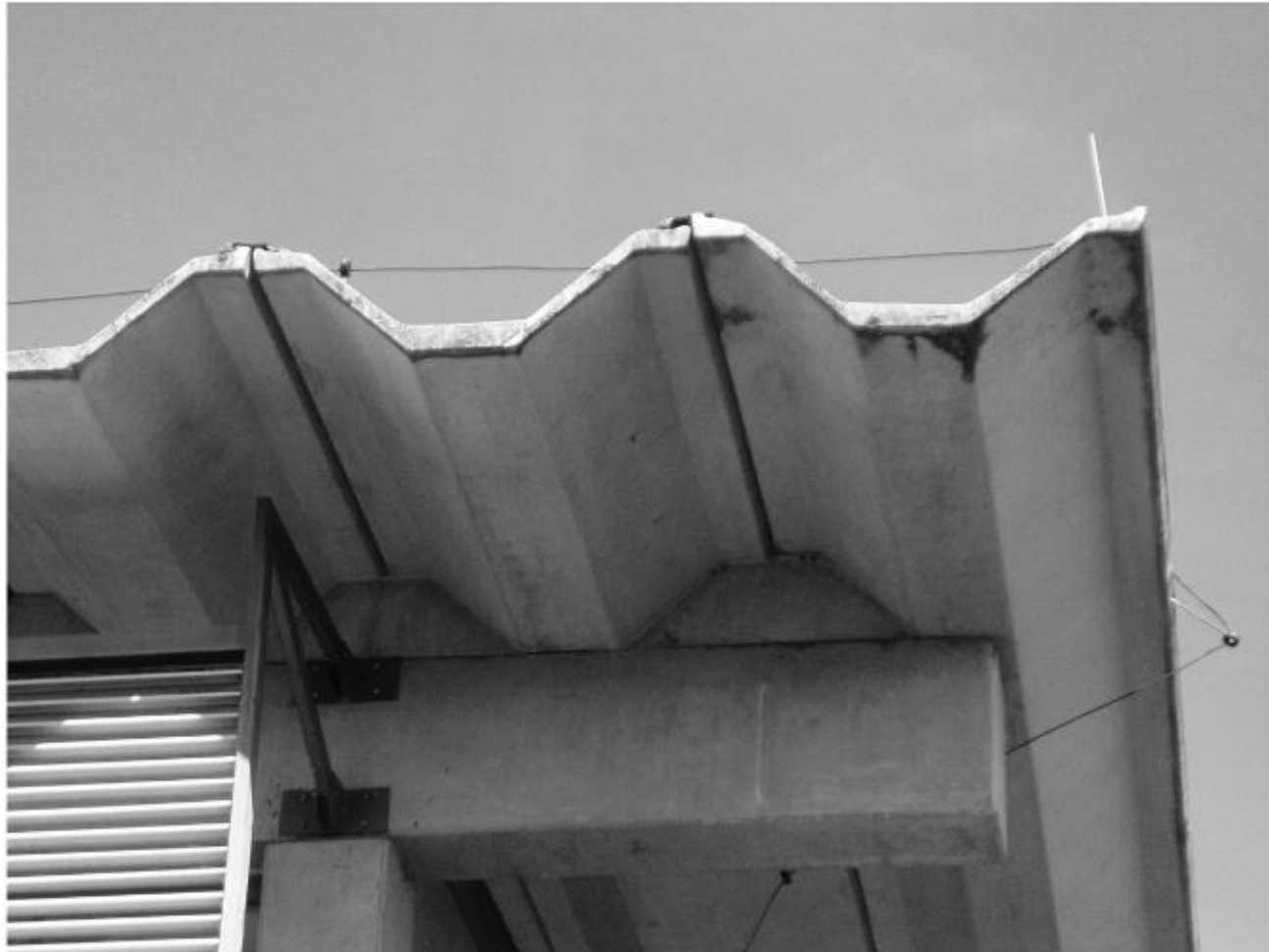
Figure 3.10 Portal frame with folded plate roof units, the University of Sao Carlos, Brazil.
