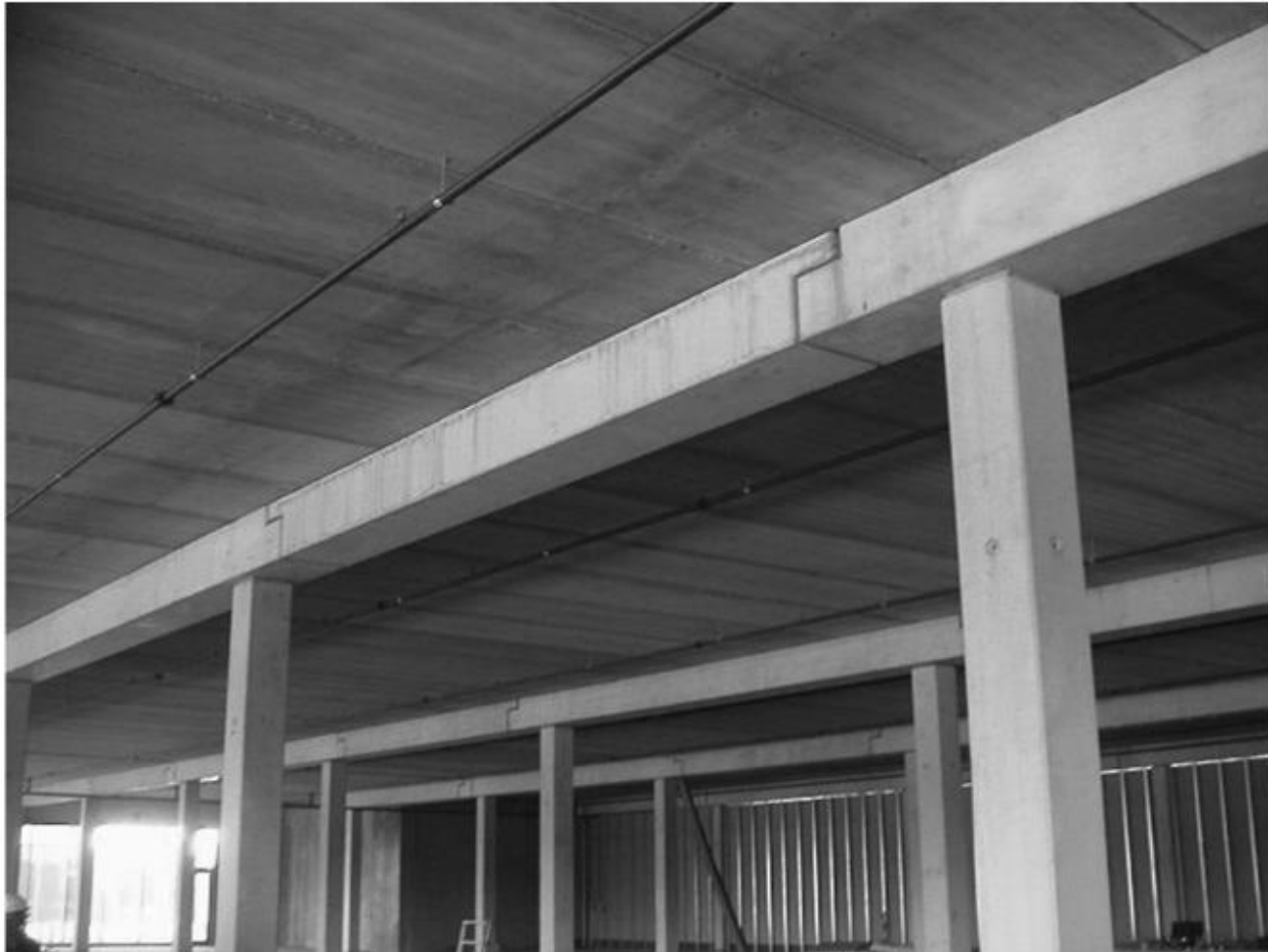
Figure 3.13 Beam half-joints at 0.1 \times span close to points of contraflexure in a continuous beam.
