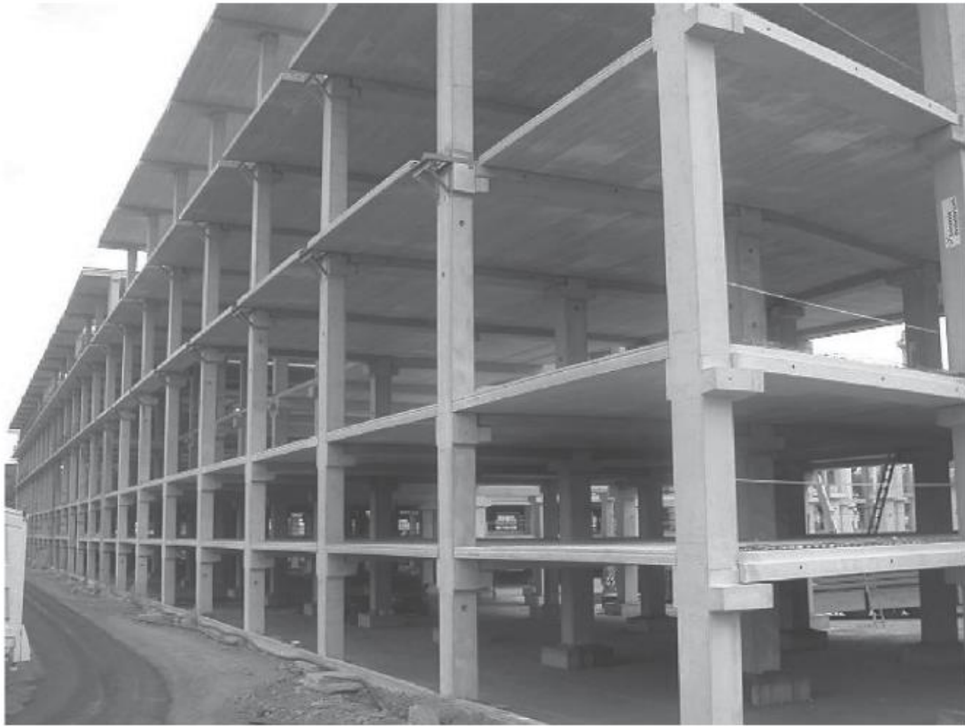
Figure 1.7 Precast concrete 'skeletal' sway frame, Europark, Rome.
