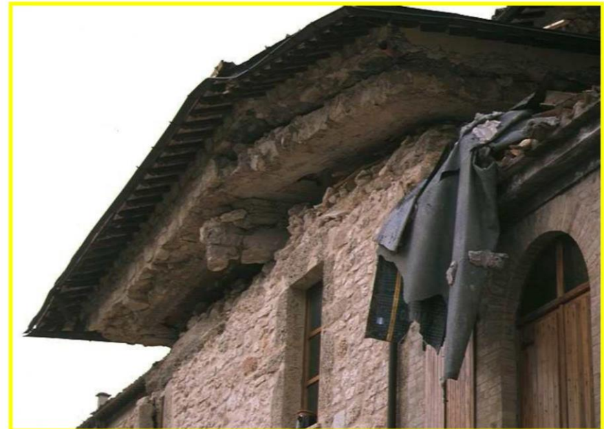
Rigid slipping of the roof
