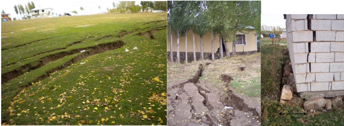
Figure. 3.2. Extensive lateral spreading due to liquefaction and resulting damages at Çelebibağı, Erciş
