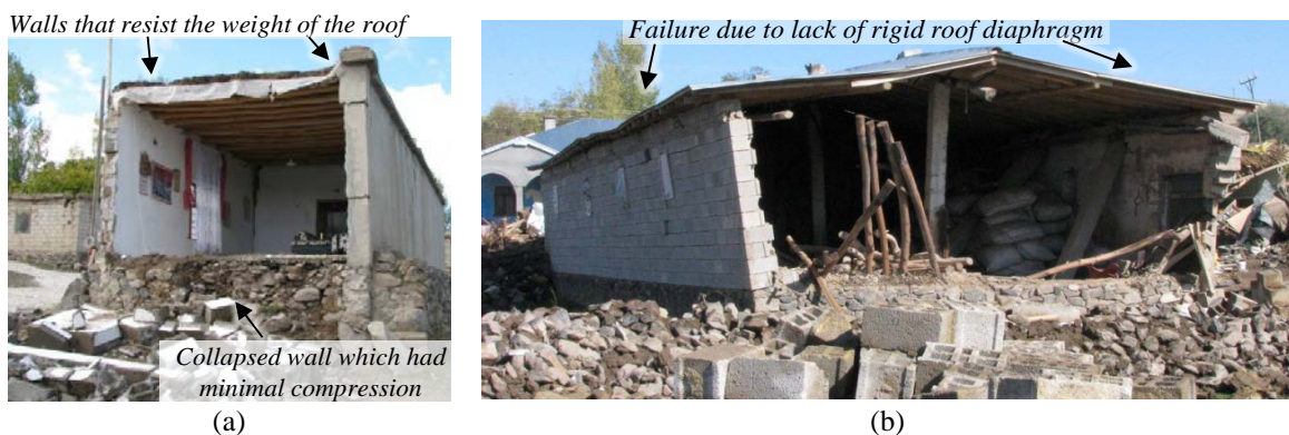
Figure 4.3. Typical damage mechanisms observed in the regional unconfined brick masonry buildings
