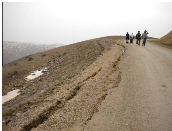
Fig. 11. Tension cracks on the side of the road in the region.
