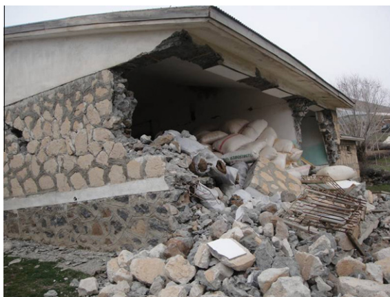
Fig. 26. Excessive wall lengths without any support or restraints and large openings ( Göçmezler village ).
