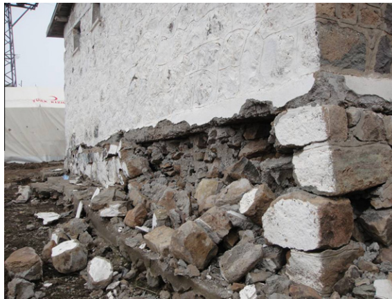
Fig. 25. Poor workmanship in the foundation ( Kayalık village ).
