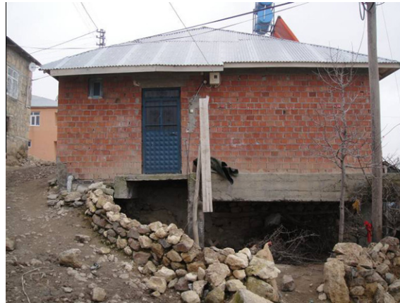
Fig. 29. Performance of an unconfined unreinforced brick masonry building (Okçular village).
