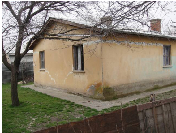
Fig. 18. Slightly damaged brick masonry buildings in Palu.
