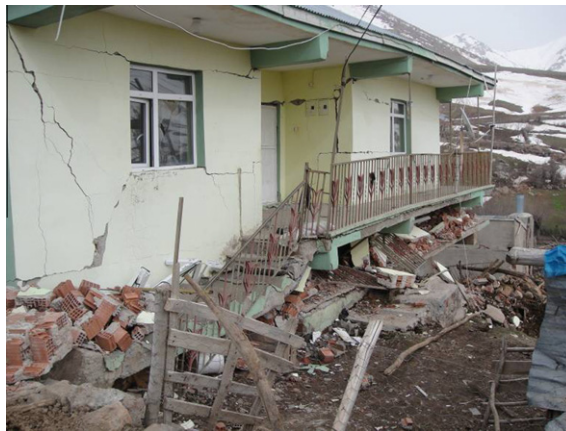
Fig. 28. Failure of a confined brick masonry building (Kayalık village).
