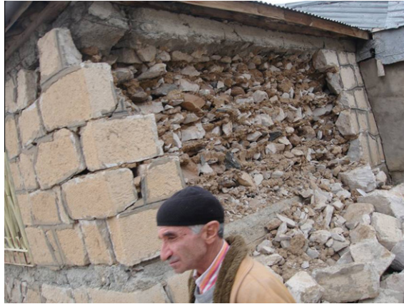
Fig. 24. Poor workmanship in wall construction, poor binder, insufficient connection in transverse direction ( Okçular village ).
