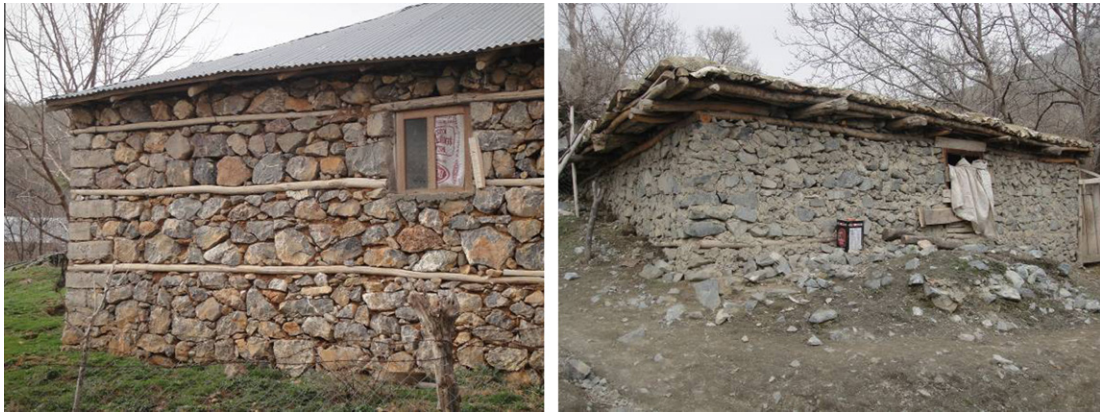
Fig. 22. Inadequate and adequate connections of walls at corners (Arındık and Köklüce villages).
