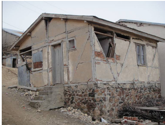
Fig. 27. Typical damage of hımiş buildings in earthquake affected region (Okçular village).
