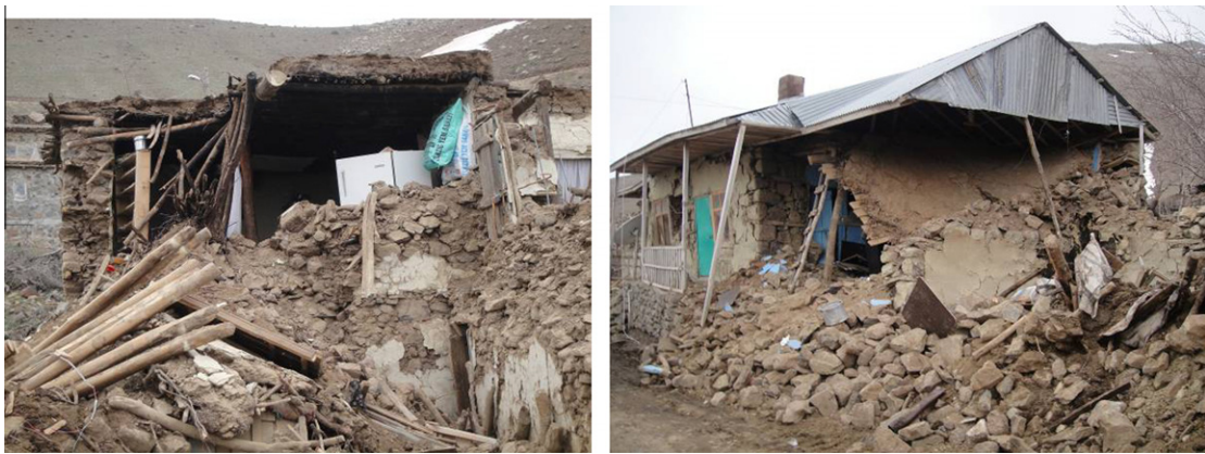
Fig. 19. Typical failures of stone masonry buildings (Göçmezler and Yukarı Demirci villages).
