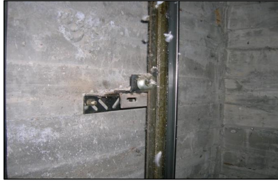
Figure 1. Damaged guide rail bracket (İmrak, 2012)
