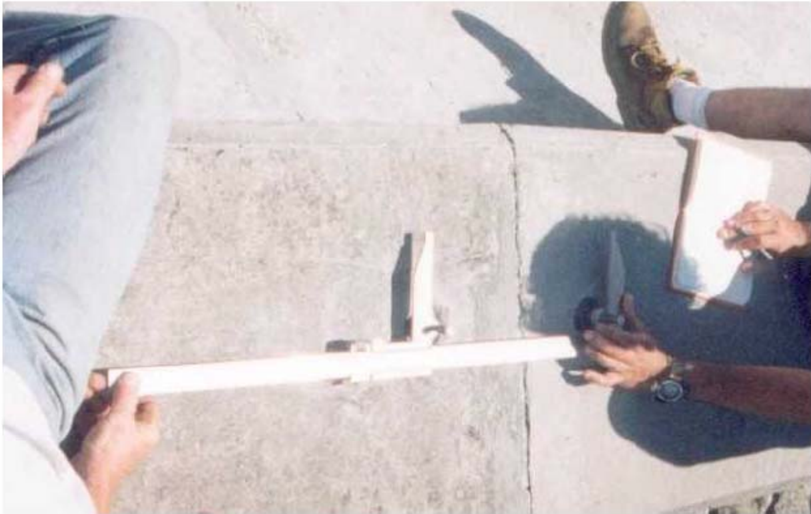
Figure 7-5. Starrett vernier caliper crack measurements between monoliths.
