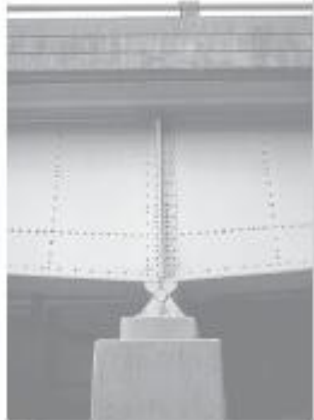
Typical pin used to support the steel girder of a railroad bridge.
