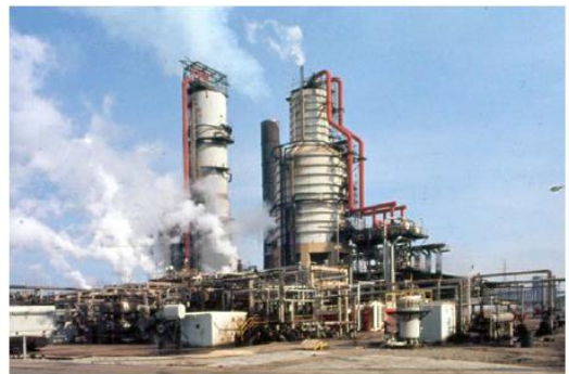
Fig. 3.5 Atmospheric and vacuum distillation units.
